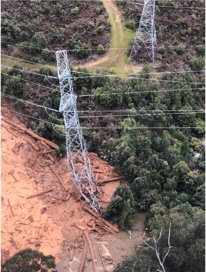
Figure 1 Double circuit strain tower damaged by landslide
