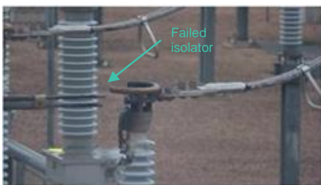
Figure 1 Isolator X31 at Buronga 220 kV substation after the incident
