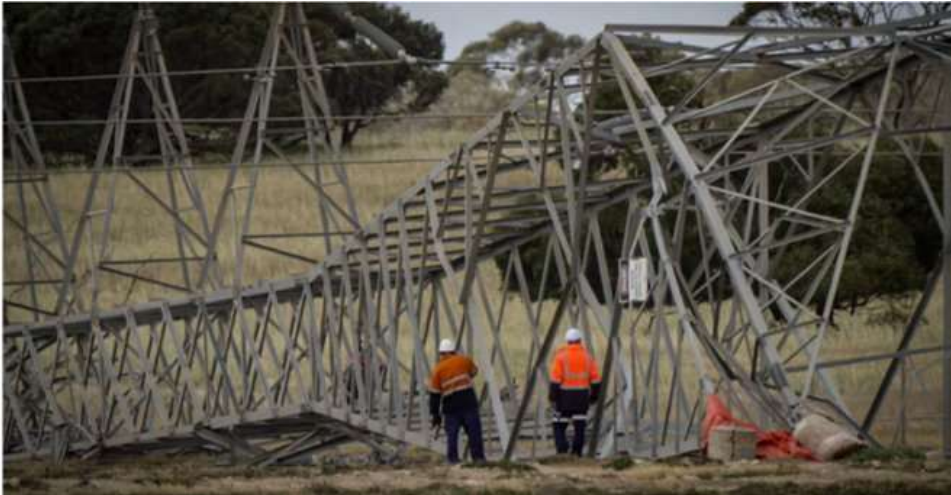
Figure 2 Photograph of the failed double circuit tower
