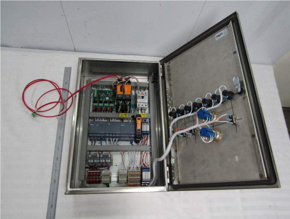
Internal view of the control cabinet
