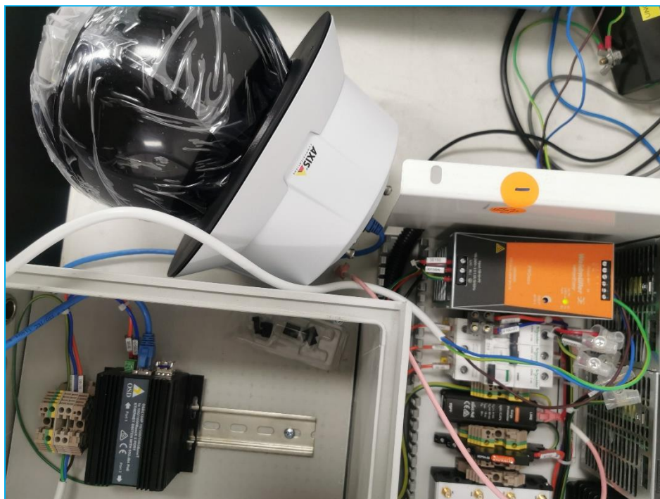
Test 3. Single power supply fed Ethernet Switch loaded with single PTZ camera.
