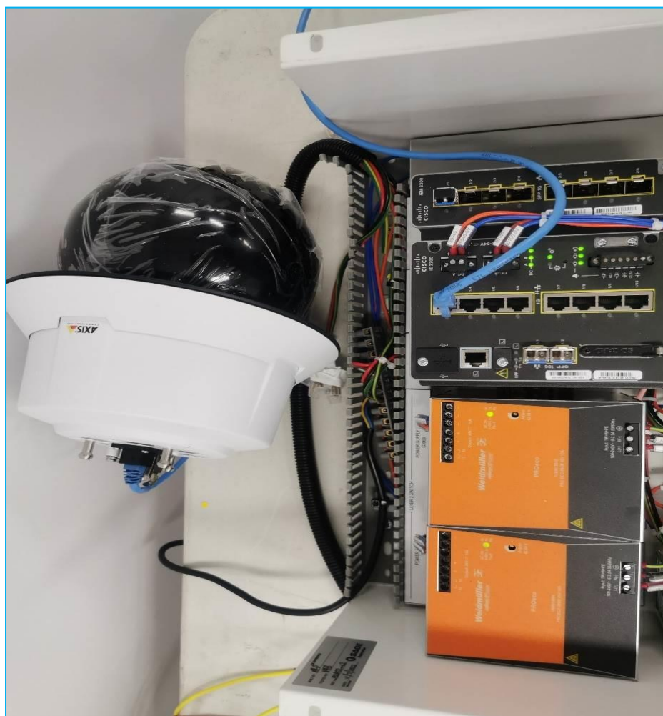
Test 4. Dual power supply fed Layer 2 Network Switch loaded with single PTZ camera
