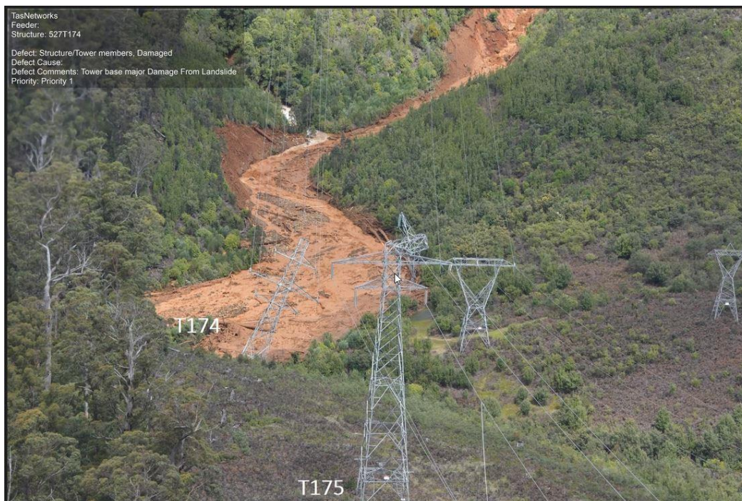
Figure 6 Damage to transmission line TL527 on 14 October 2022 due to a landslide event
