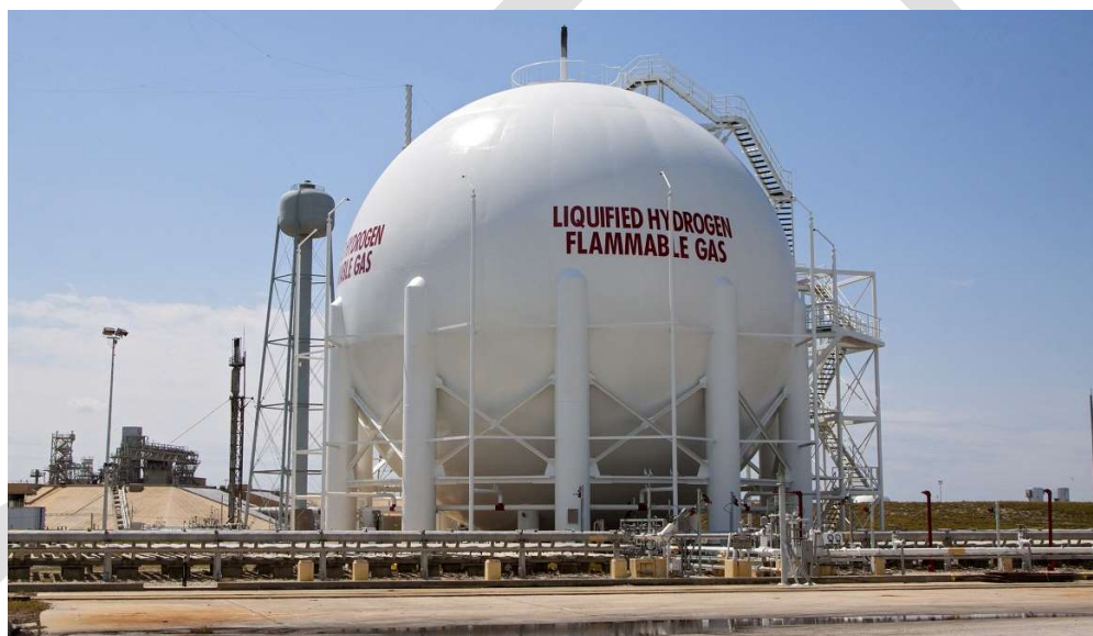
Figure 5-1: Hydrogen storage tank, Cape Canaveral (picture NASA)
