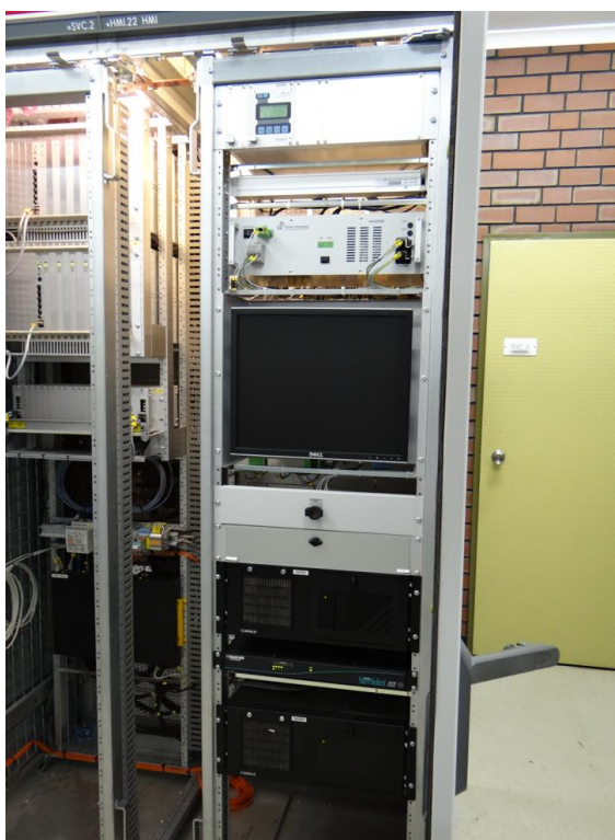
Figure 2 – SVC 2 secondary system cabinet including computer control system
