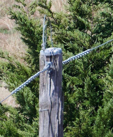
Figure 2-4 Wood pole deterioration
