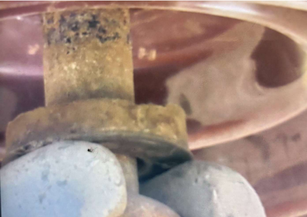
Figure 2-3 Deterioration of insulators
